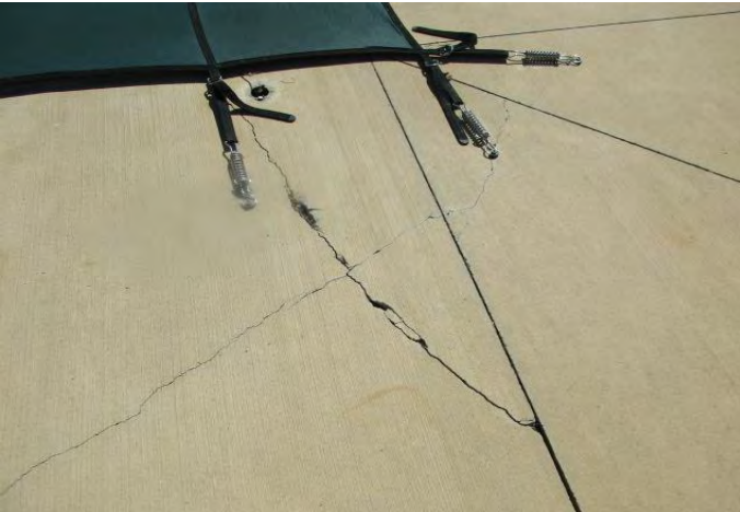
Cracks at concrete pool deck
