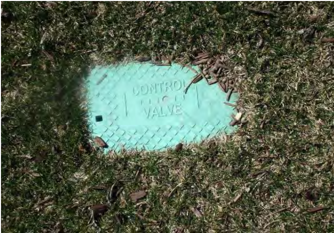
Irrigation control valve near clubhouse
