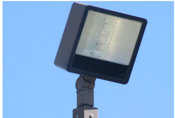
Typical light fixture at swimming pool
