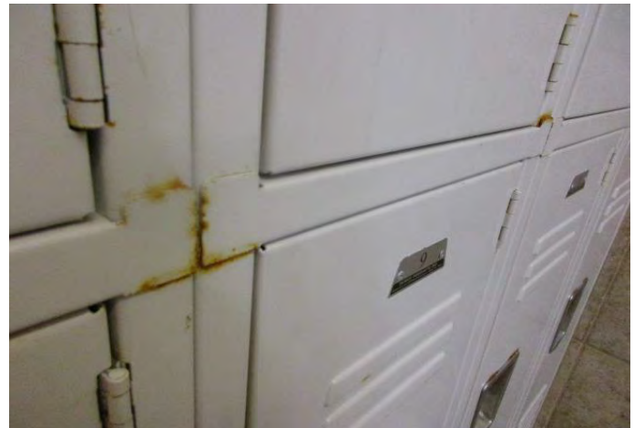
Rust at metal lockers at restroom
