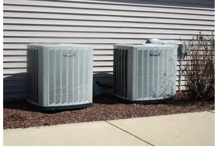
Exterior condensing units at clubhouse
