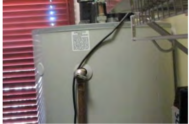
75-gallon water heater
