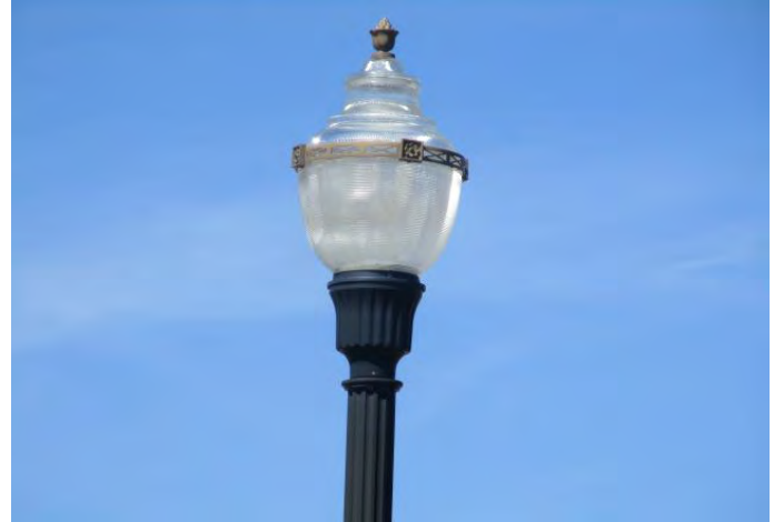
Typical light fixture at parking lot
