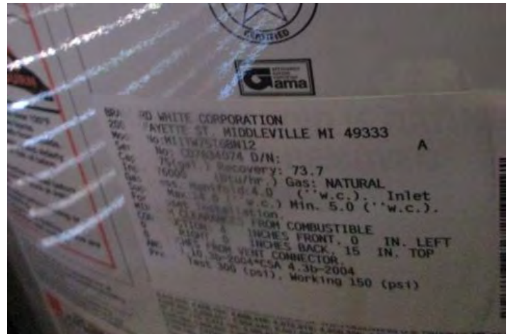
Specification tag at water heater
