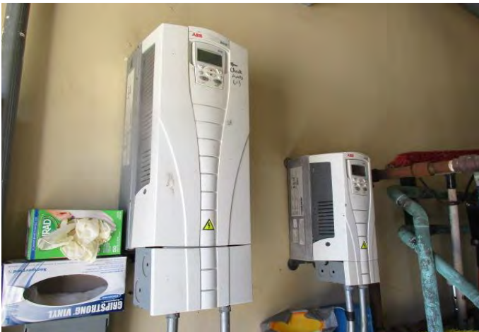
Variable frequency drives for pool pumps
