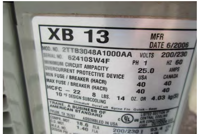
Specification tag at condensing unit
