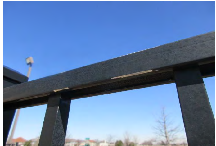
Condition of chipped finishes at top fence rail
