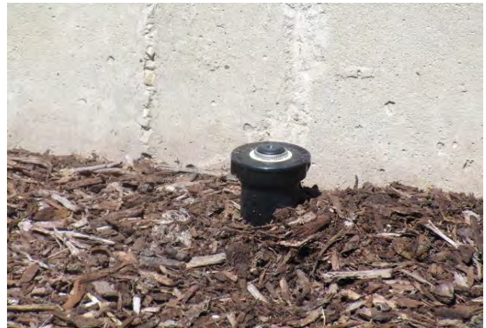
Irrigation head at planting bed
