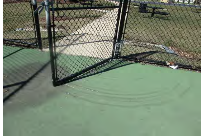
Worn coloring / markings at gated entrance
