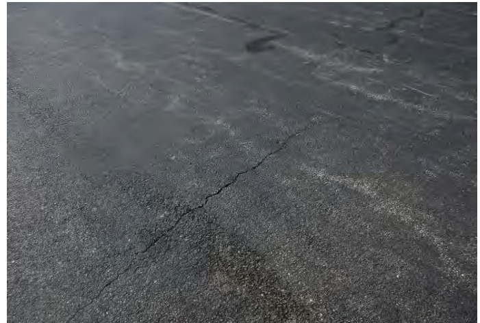
Cracks at asphalt pavement
