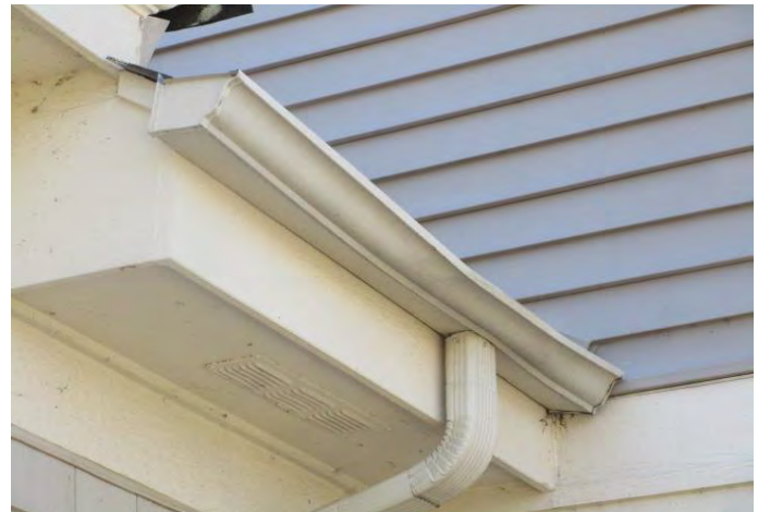
Dented aluminum gutter at roof eave
