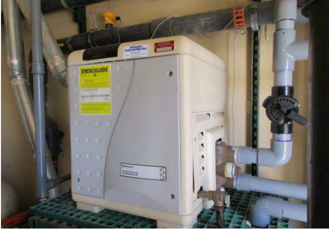
Heater for swimming pool
