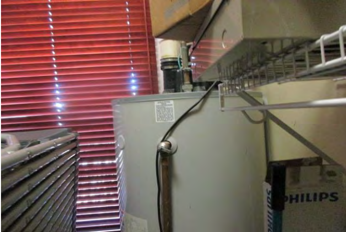
Water heater at clubhouse mechanical room
