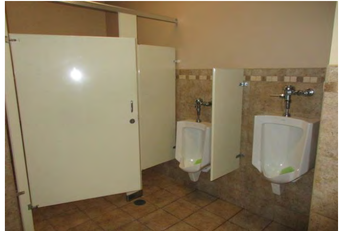
Men's restroom fixtures and partitions
