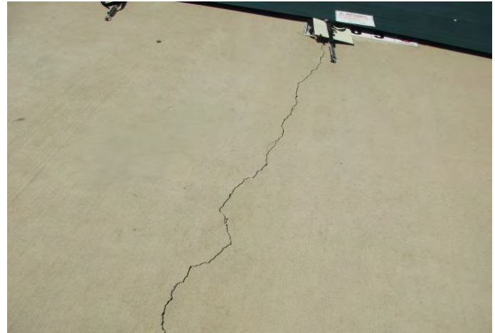
Cracks at concrete pool deck
