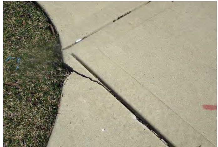
Crack at sidewalk, near control joint
