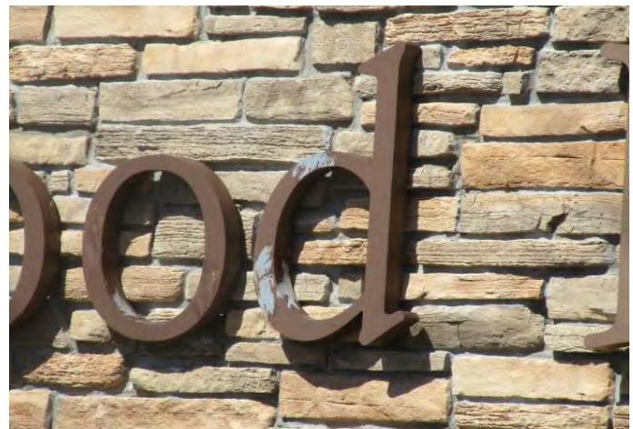
Chipped finishes at metal lettering at south property entrance
