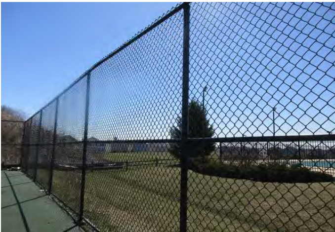
Typical condition of vinyl-coated fencing
