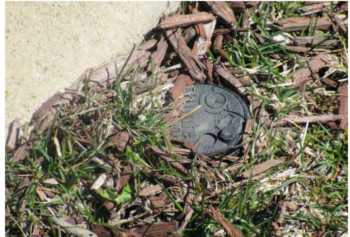
Irrigation head at lawn area
