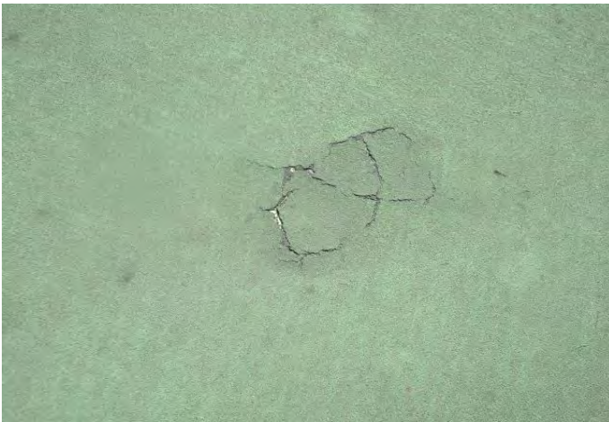
Cracks and depression at court surface
